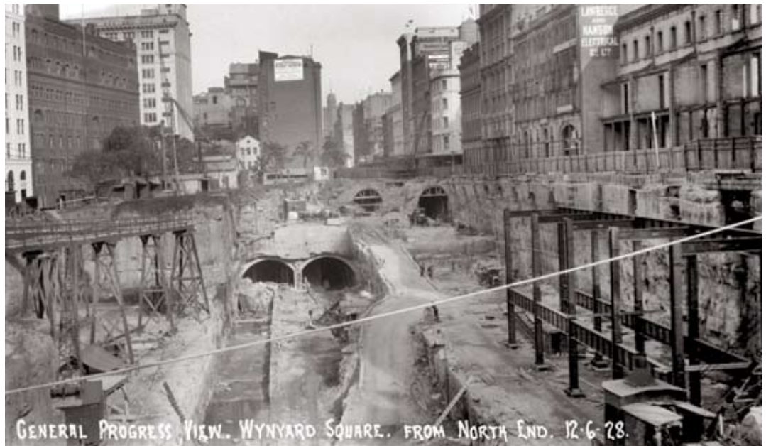
General progress view, Wynyard Square, R C Roberston, 1928, printed from glass plate negative, State Records NSW
