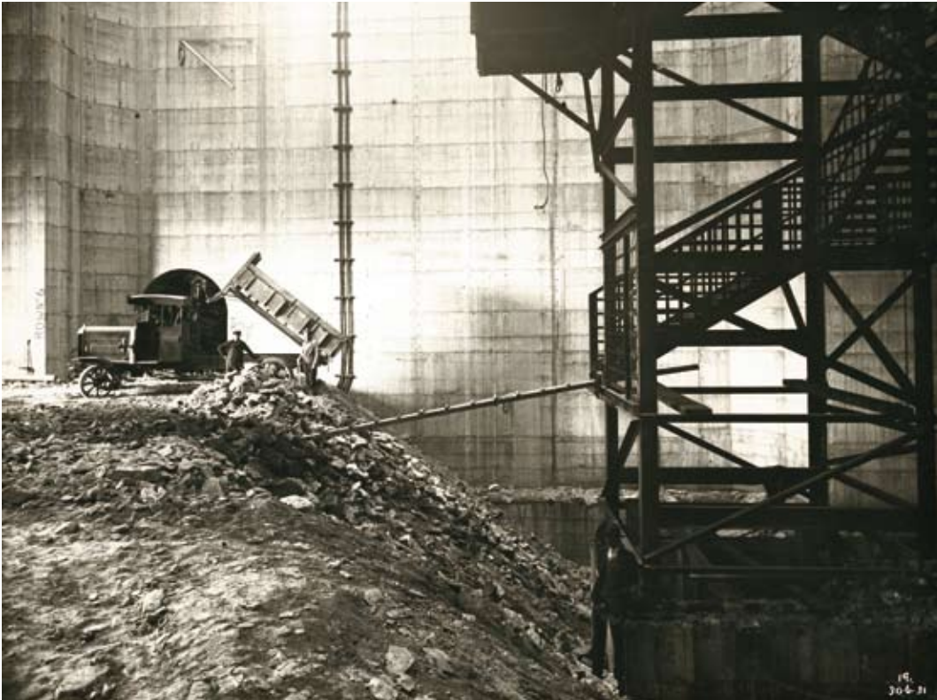
Levelling floor of pylon , photographer unknown, 30 June 1931, Sydney Harbour Bridge Photographic Albums 1923–1933, vol 8, State Records NSW
